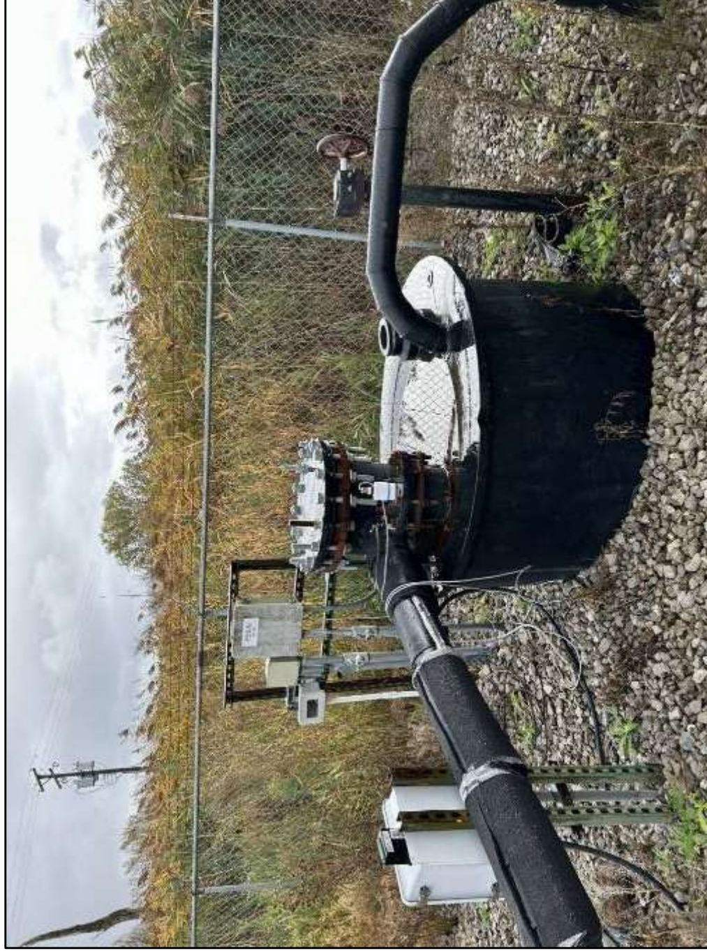
Main Condensate Knockout and Pump Station Vessel.
